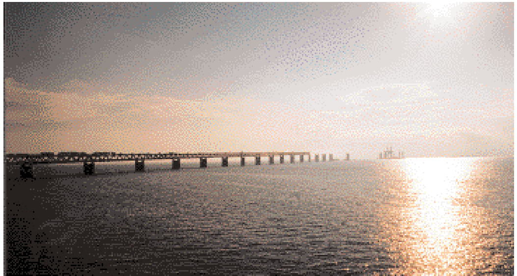
At the moment, the high-level bridge emerges from the Øresund like a deep-sea oil-drilling rig. The shore spans of the bridge advance from the Swedish coast with a giant's steps.
