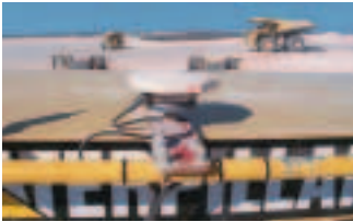
The Rover GPS radio receiver is mounted on top of the Dozer.
