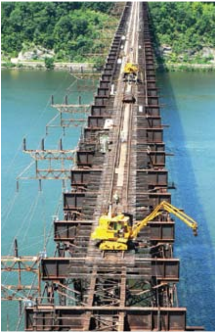
Above: An aerial shot of the bridge before the renovation work began.
