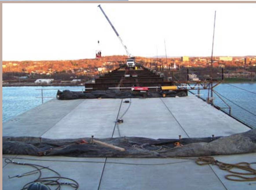
Left: Adolf Jonietz locates points on the curve of the east approach of the bridge. Above: Massive concrete panels are set in place for the new walkway.
